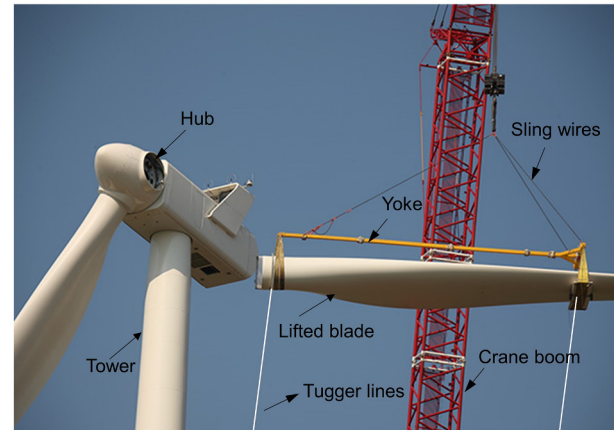
Fig. 2. Image of a wind turbine blade being prepared to mate with hub of a turbine (source: [13]).
